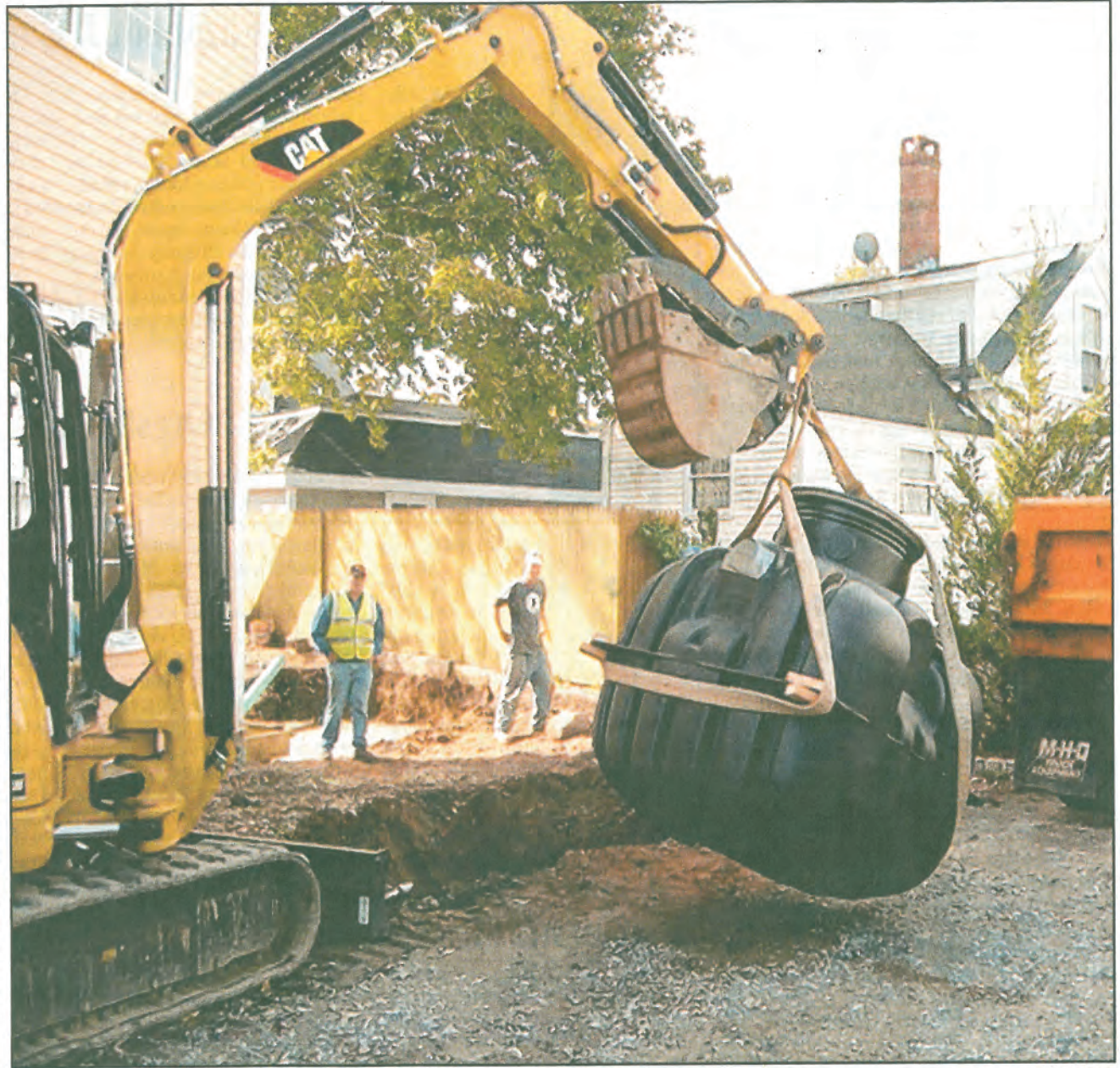
A large storage tank was recently installed at the Rockport Community House to harvest rainwater for use in irrigation.
